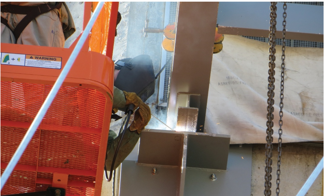
A welder performing shielded metal arc welding attaches a platform frame to a steel base plate at Calvert Cliffs Nuclear Power Plant, Lusby, Md. (Photo courtesy of Glenn R. Frazee.)
